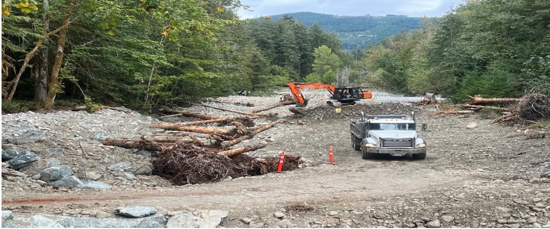
By mid September LWD was anchored in place and last of the many loads of excess gravel were removed.
