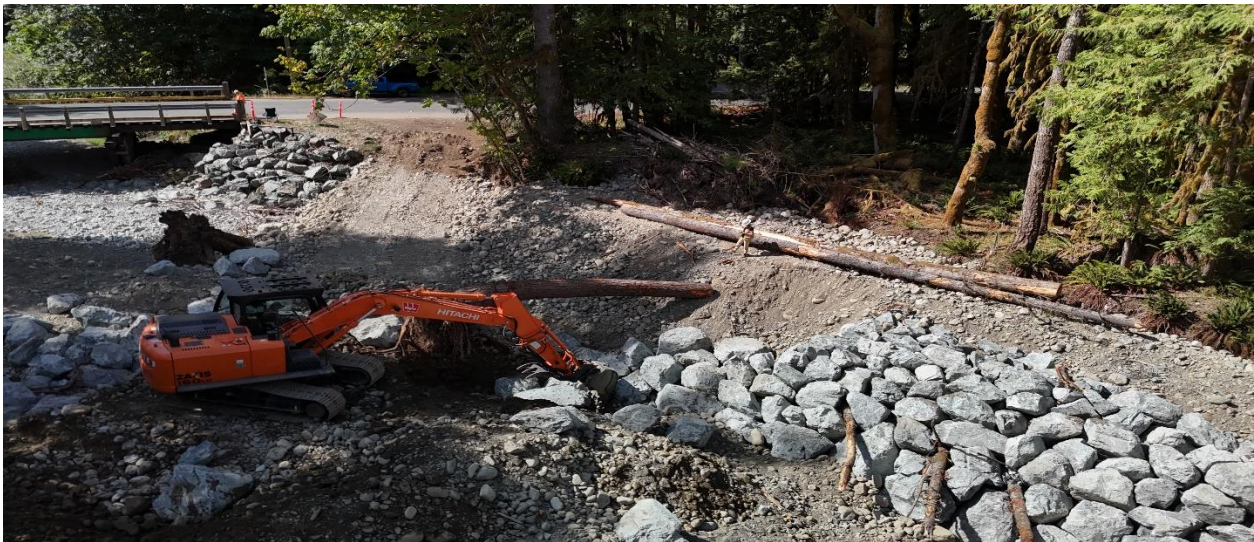
Keying in dry blasted rock boulders for armoring against hydraulic stream forces. Drone Photo Ernest Pilfold.
