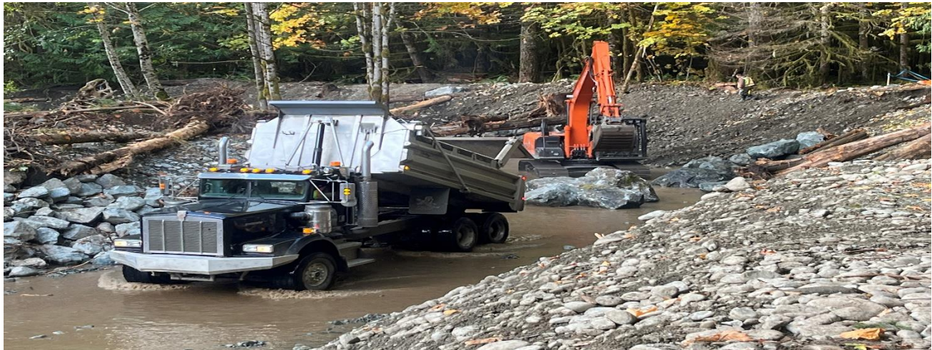
Deliveries of large, blasted rock boulders arriving for anchoring LWD and habitat enhancement.
