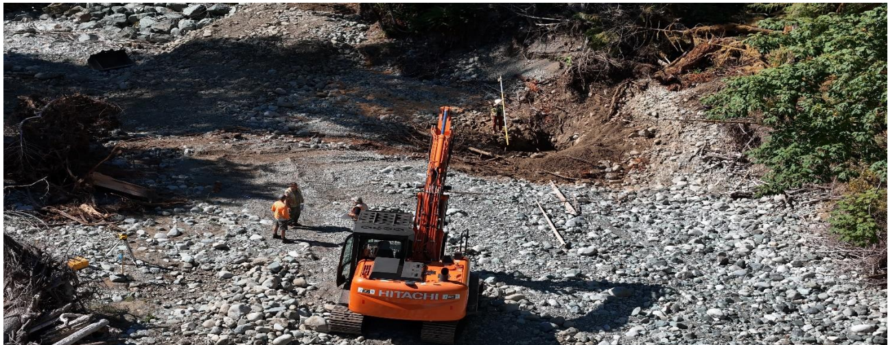
Locating elevation of water table is an important first step for constructing scour pools for fish habitat. MOTI Surveyor Kiara Smith runs elevations. (Drone photo Ernest Pilfold).
