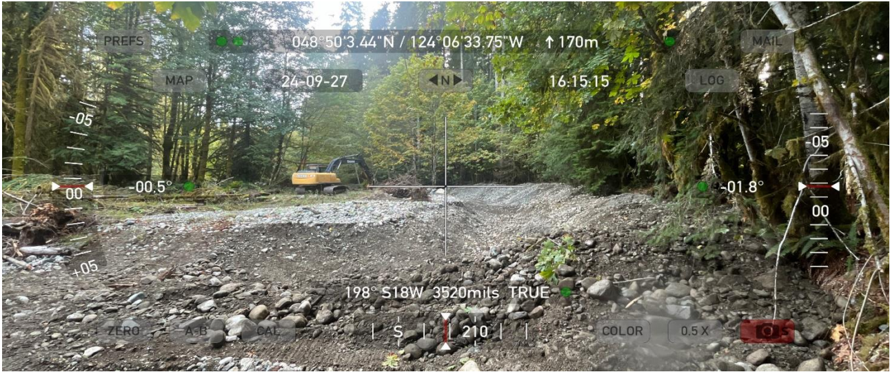
Late in September Phase II has started downstream of Meade Creek Road bridge on the Mac Rae property.
