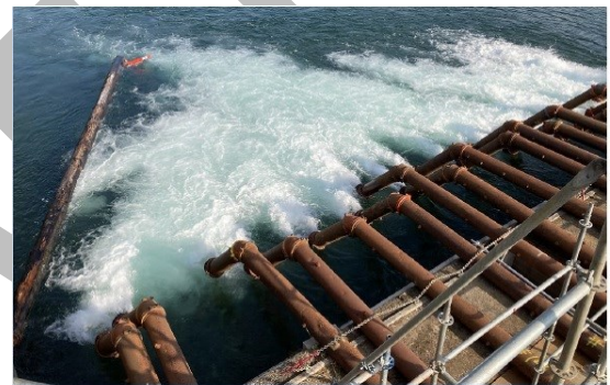
PUMPING WATER OVER COWICHAN WEIR TO KEEP THE RIVER FLOWING. 2023 (PHOTO COURTESY OF CATALYST PAPER)
