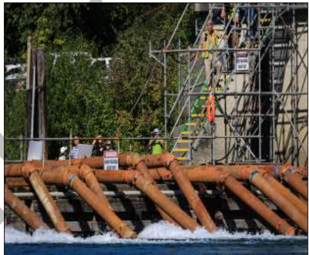
Electric pumps keeping the Cowichan River flowing.
